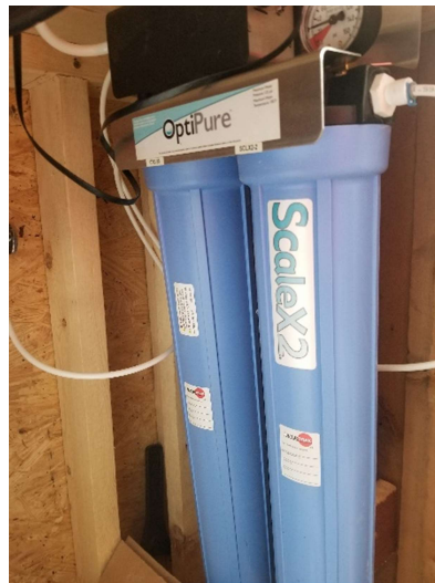
Figure 4. Water filtration equipment for espresso machine.
